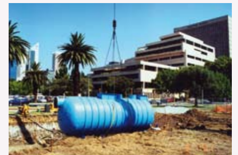
SPEL STORMCEPTOR™ treating stormwater from various carpark and streets in PERTH CBD - Perth City Council.
