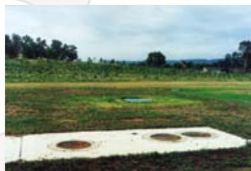
SCOPES CREEK, PENRITH CITY COUNCIL, NSW. - Wood lot in the background is irrigated by the treated water by the STORMCEPTOR™.
